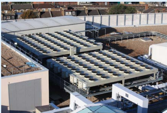
61 Güntner GFH drycoolers ensure low-noise and energy-efficient operation at Westfield London.
