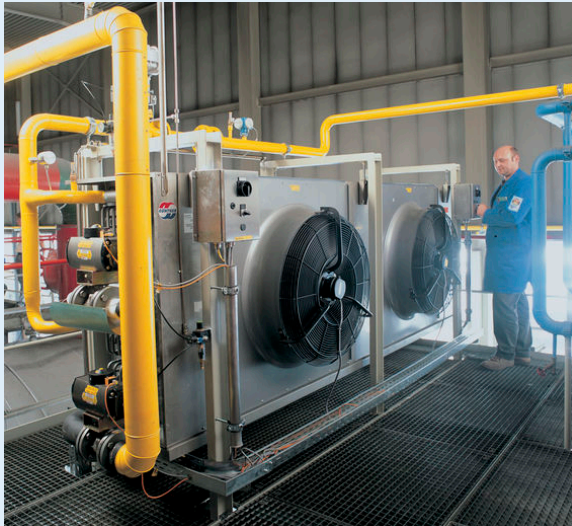
Güntner GPN CO 2 process evaporator in use at Paulaner brewery
