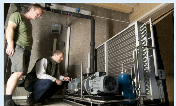
Brewery owner Robert Neumaier (left) and chiller manufacturer Karl Huber (right) assessing the quietness of the glycol brine chiller. To improve the air flow and further reduce noise, the space between the condenser and the opening in the outer wall was also enclosed.
